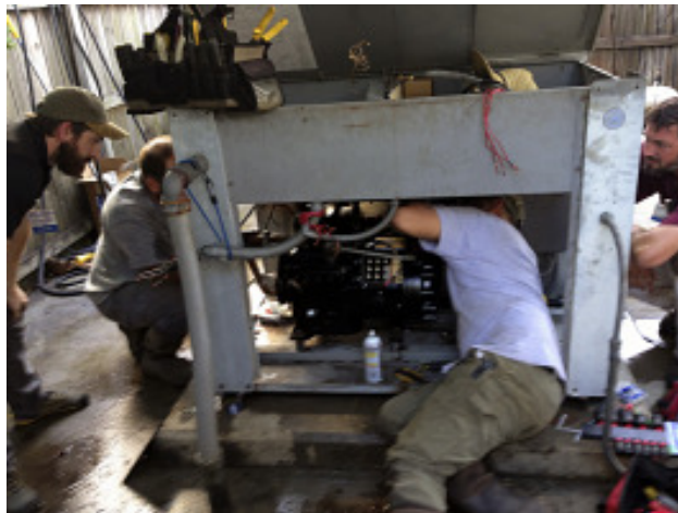
Properties staff attempt to revive an old air-conditioning system in the Pediatric Care Center. Two of the department’s associates even drove to Birmingham to pick up a pump/compressor that could not be found locally.
